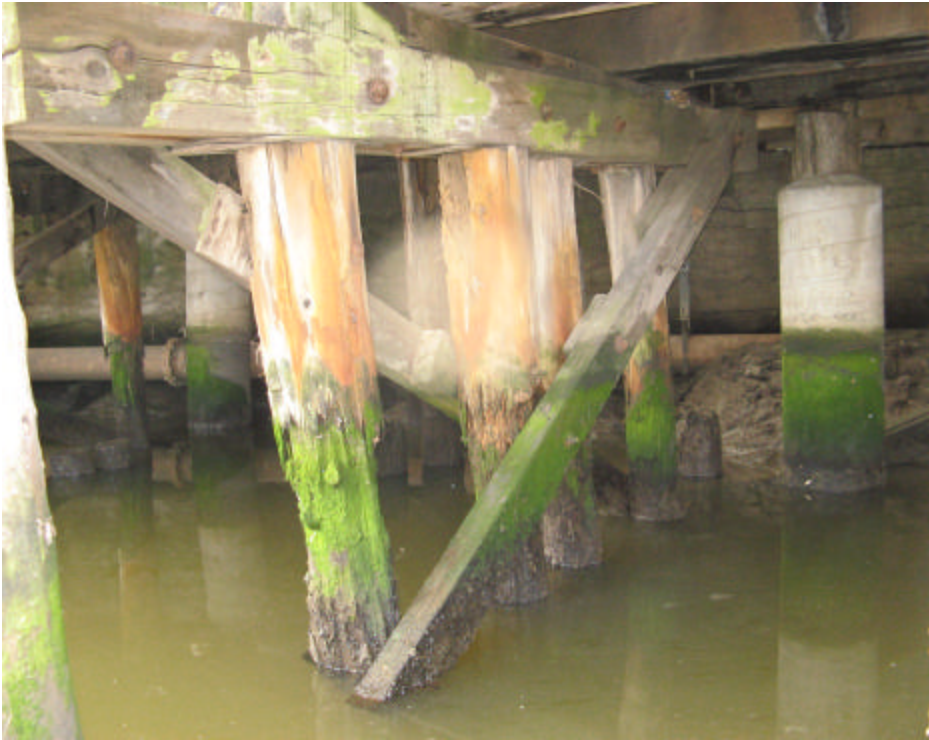
Figure 5: Typical Pile Cross Section Loss – Bent 6 (nearest pile rated “fair”) Beyond the bent is a concrete pile associated with the deck adjacent the Mill building. Bent 6 is a four-pile bent.
