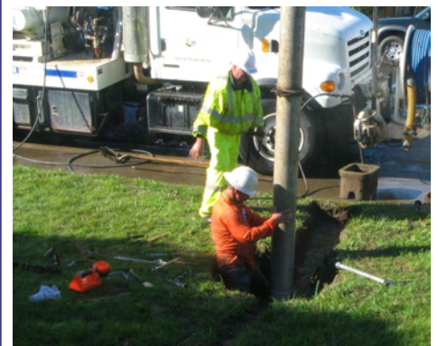
Water team repairs a 6-inch water line near Middlefield Drive. The Water Dept. completed over 240 water line repairs this year, which is much higher than the national average.
