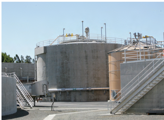
Large tanks at the Ellis Creek Water Recycling Facility called digesters breakdown and treat waste material.
