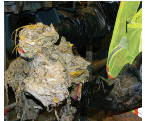
Maintenance crew removing wipes from clogged pumps.
