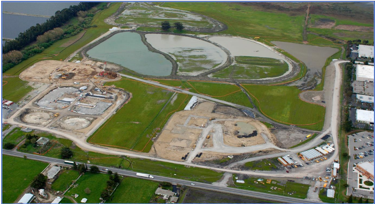
This is an aerial shot of early construction on the City's new $140 million sewer treatment plant.
