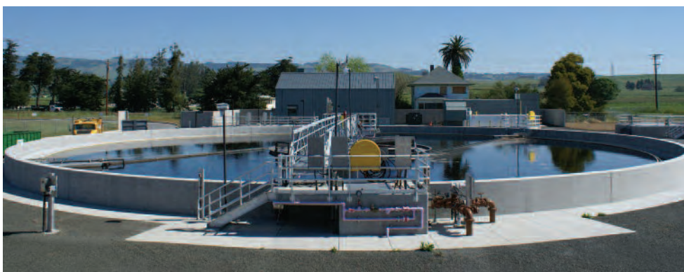
Photo of secondary clarifier which began cleaning Petaluma's wastewater on January 6.
